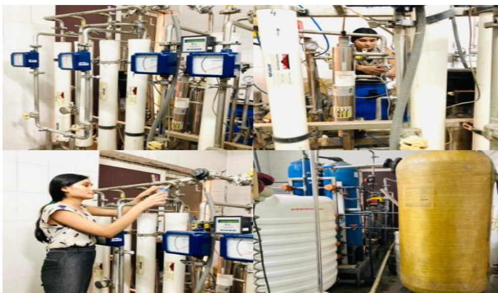
Figure 9 NEW WATER PLANT
