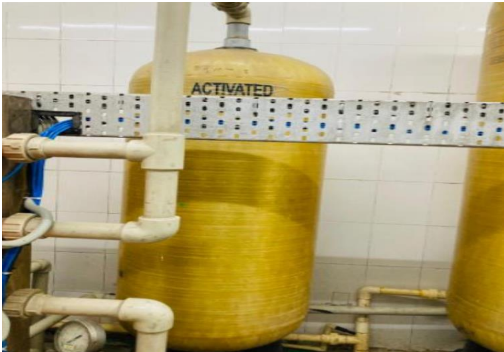
Figure 3 Activated Carbon Filter
