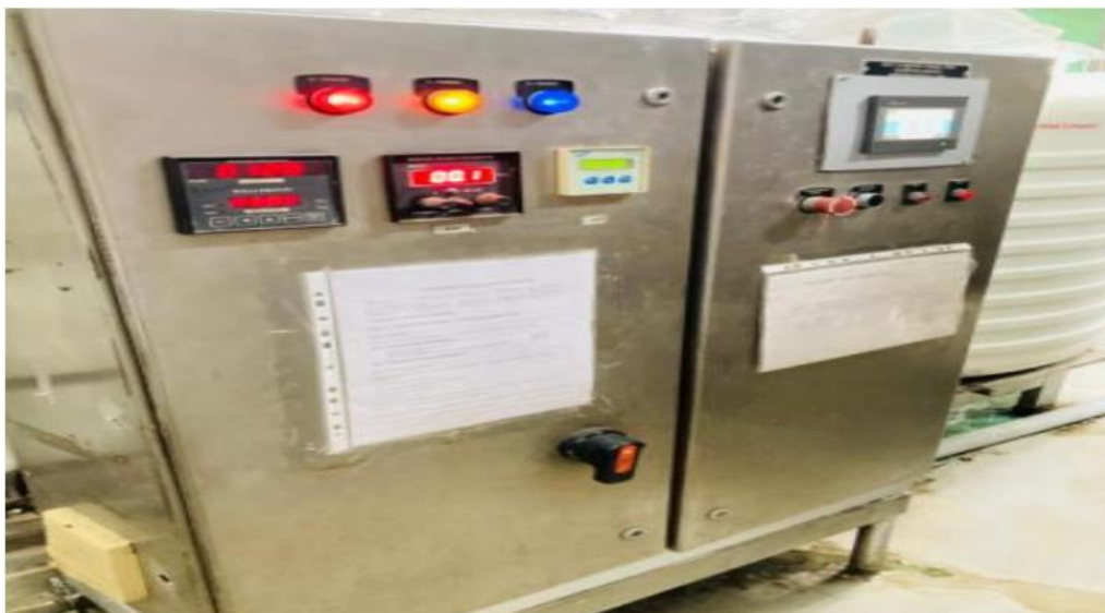
Figure 10 CONTROL PANEL OF NEW WATER PLANT
