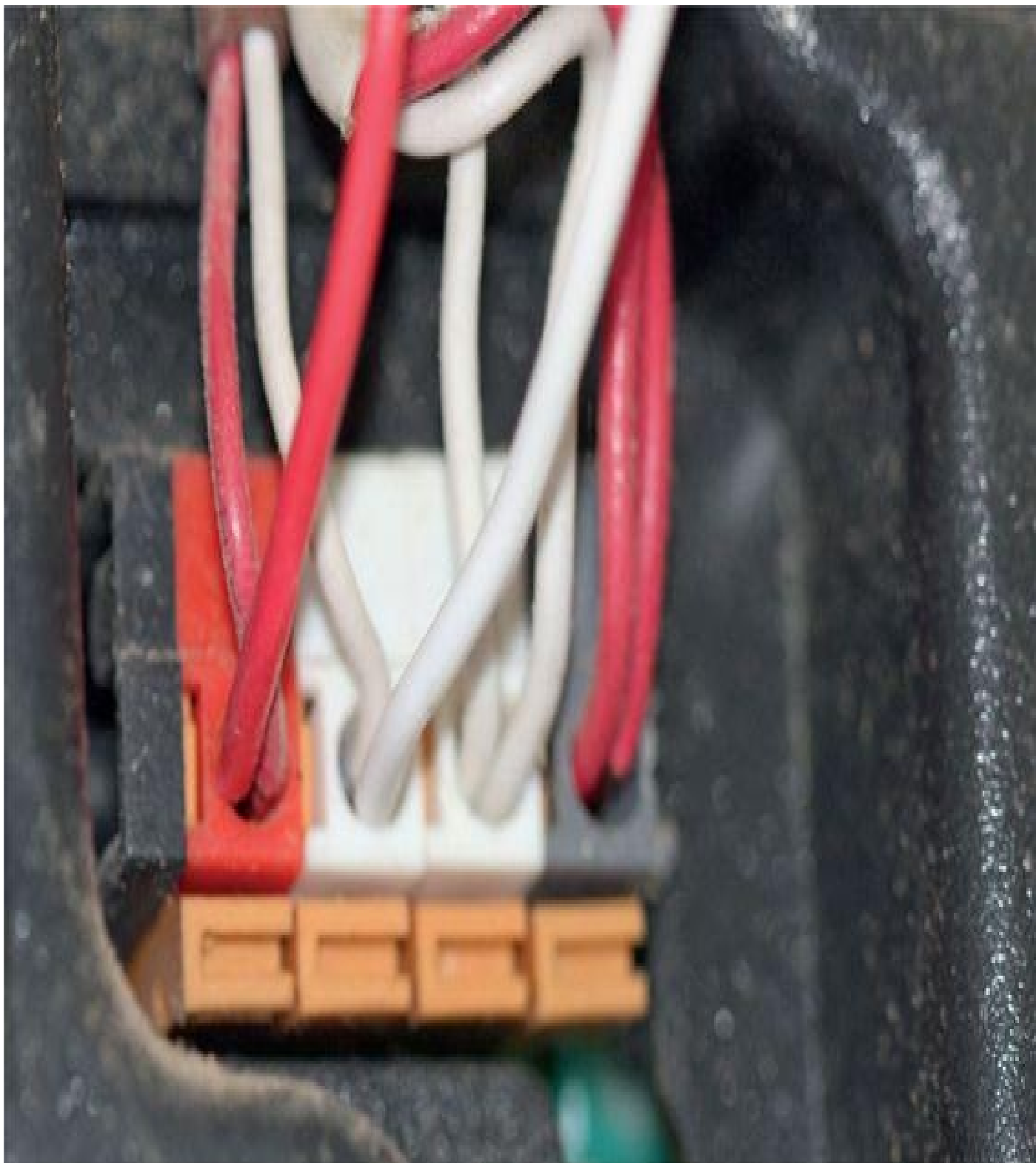
FIGURE 6-15 Garage door opener connection terminals
