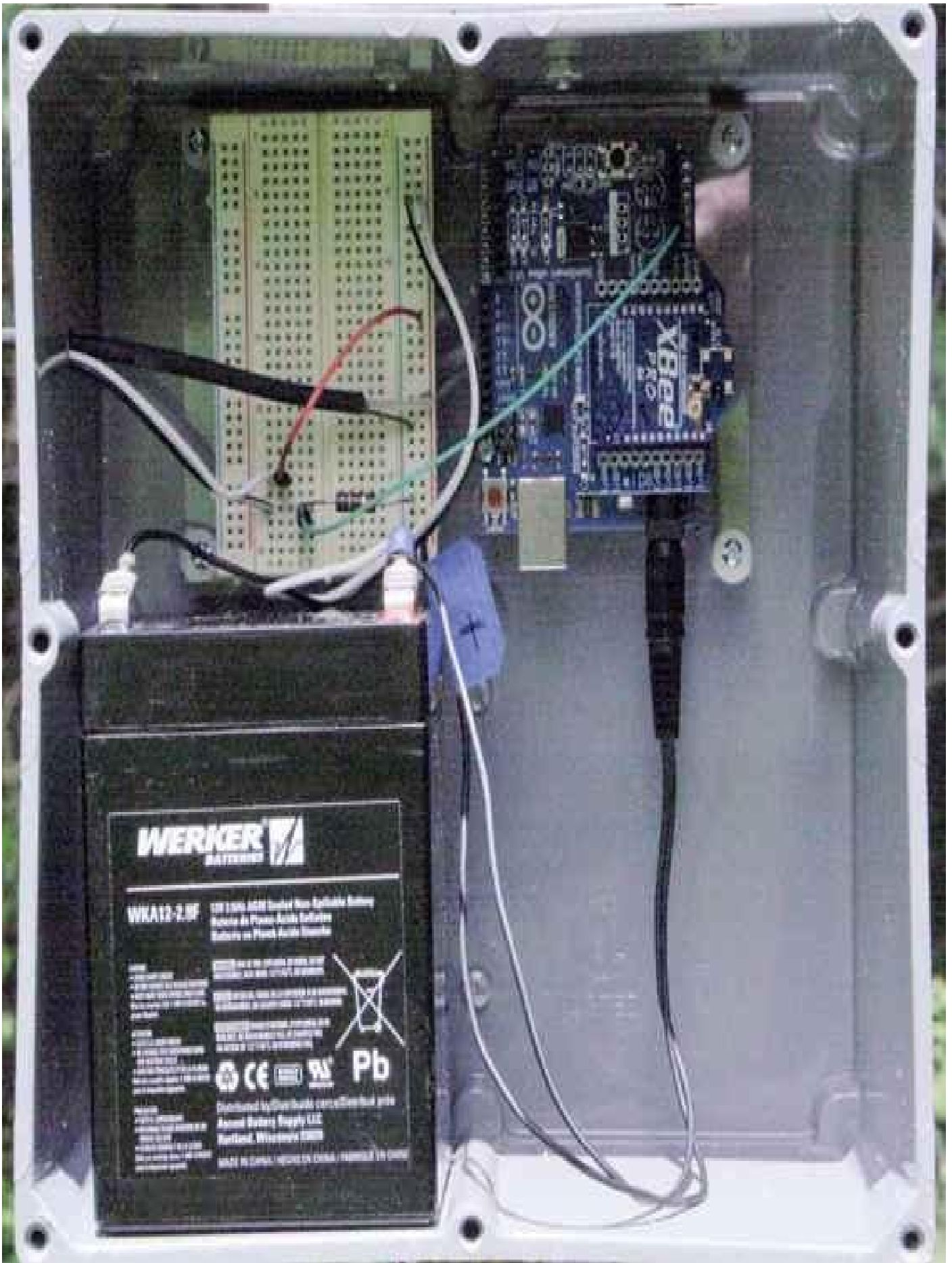
FIGURE 7-22 Interior of the moisture system enclosure
