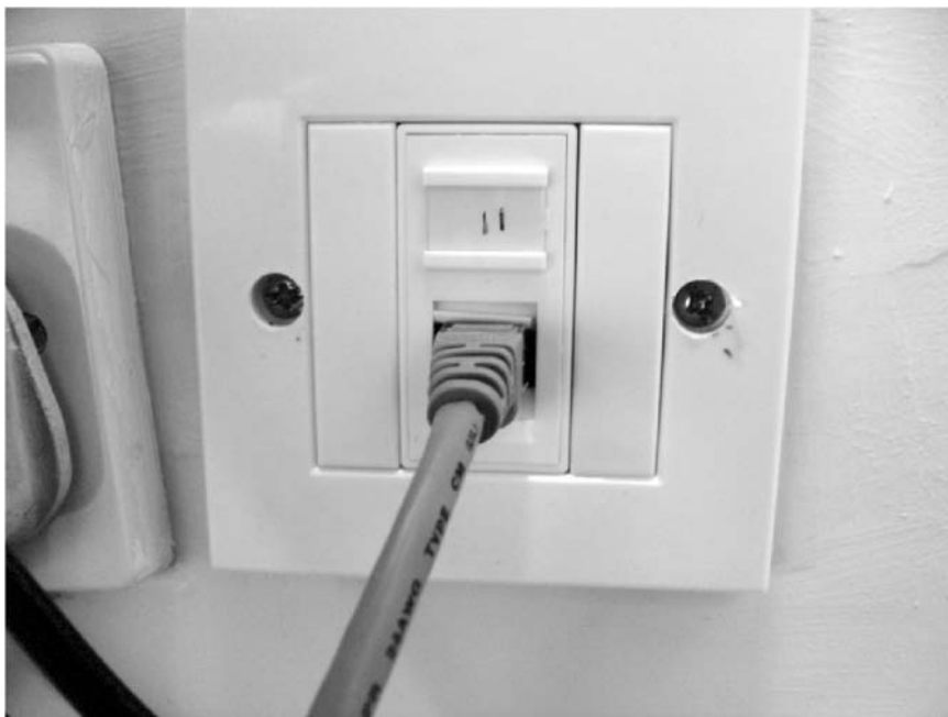
Figure 3.13 A standard RJ45 wall plate in the author's bedroom
