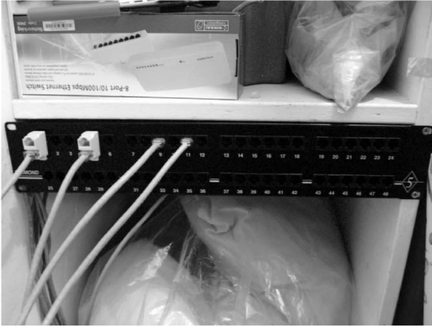
Figure 3.14 A network patch-panel in a domestic installation
