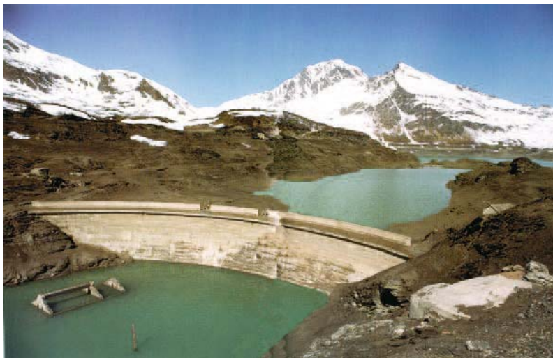
Fig. 103. The old MONCENISIO dam emerges out of the waters of the new reservoir [44]
