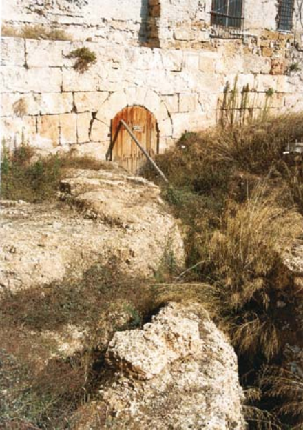
Fig. 17. The bottom outlet of the Mare Dolce pond (photo by C. Gambino, 2002)
