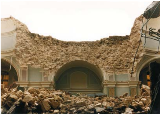
Fig. 42. The soft calcarenite placed in a random fashion in the masonry of the San Corrado church at Noto which failed without premonitory evidence in March of 1996 (photo by V. Jappelli, 1996)
