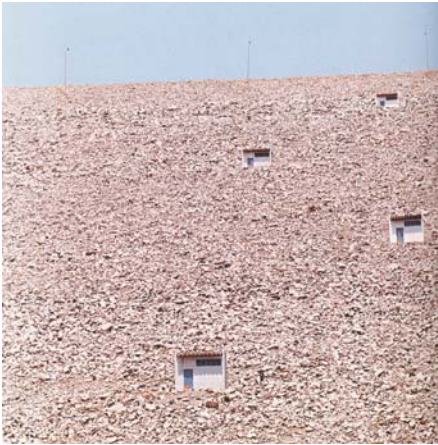
Fig. 54. Windows for the instruments on the downstream slope of a rockfill dam [34]
