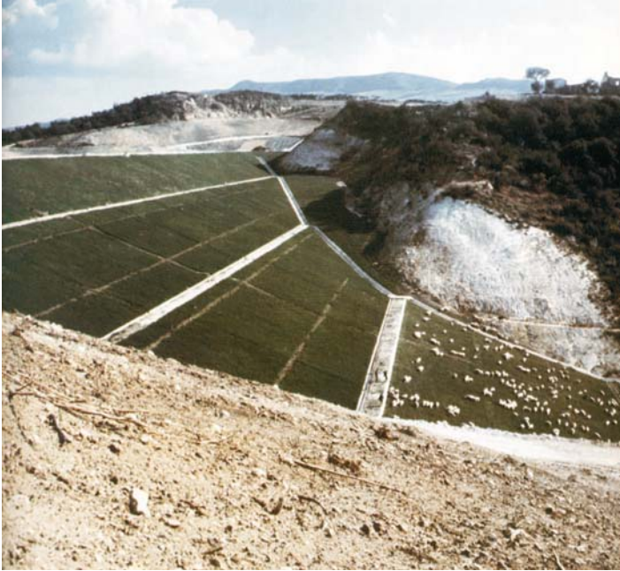
Fig. 68. The downstream slope of the POMA embankment dam on the Iato River near Palermo, Sicily; a flock of sheep graze on the grassy dam facing [6]
