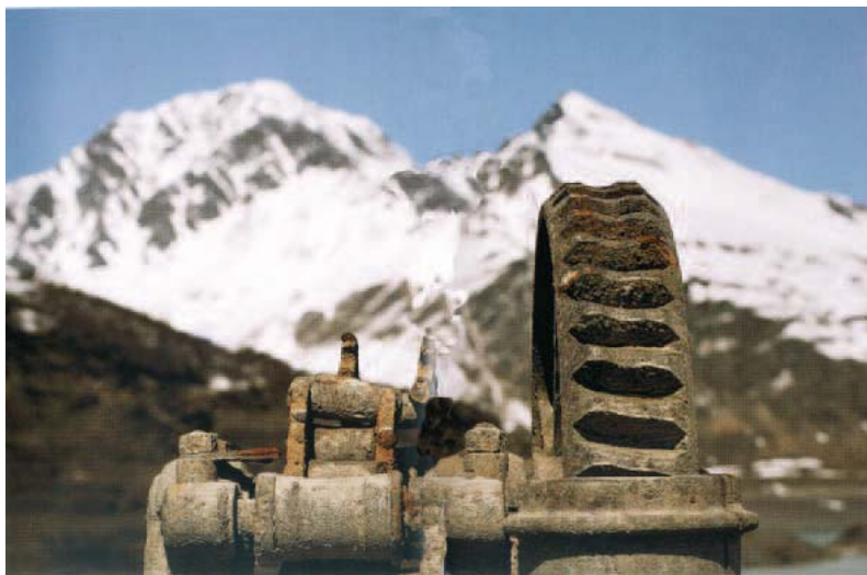
Fig. 105. Views of the territory around the MONCENISIO reservoir on the occasion of a drawdown; devices for the lifting of old gates from the Savigliano Workshops [44]
