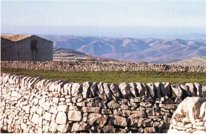
Fig. 73. The elementary dry masonry walls dividing the property in the Iblean plateau
