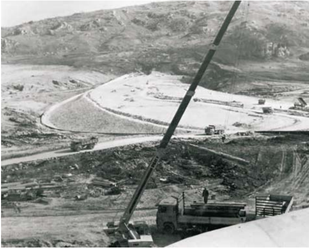
Fig. 38. The left abutment of the CASTELLO embankment dam near Agrigento (Sicily) rests on a large, stabilized landslide
