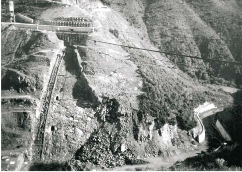
Fig. 100. The work at the ALTO ESARO near Cosenza, Italy, was interrupted in 1987 in consequence of a rupture with a mechanism in the rock formation during the excavation at the left abutment of the concrete gravity dam ( H = 120\text{ m} ) [10]
