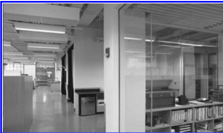
FIGURE 13.9 Heated and chilled beams in an office. (From Massachusetts Institute of Technology, Chilled Beams Hit the Roof , Cambridge, Massachusetts, Accessed on December 19, 2014, http://mitei.mit.edu/news/chilled-beams-hit-roof , 2009.)
