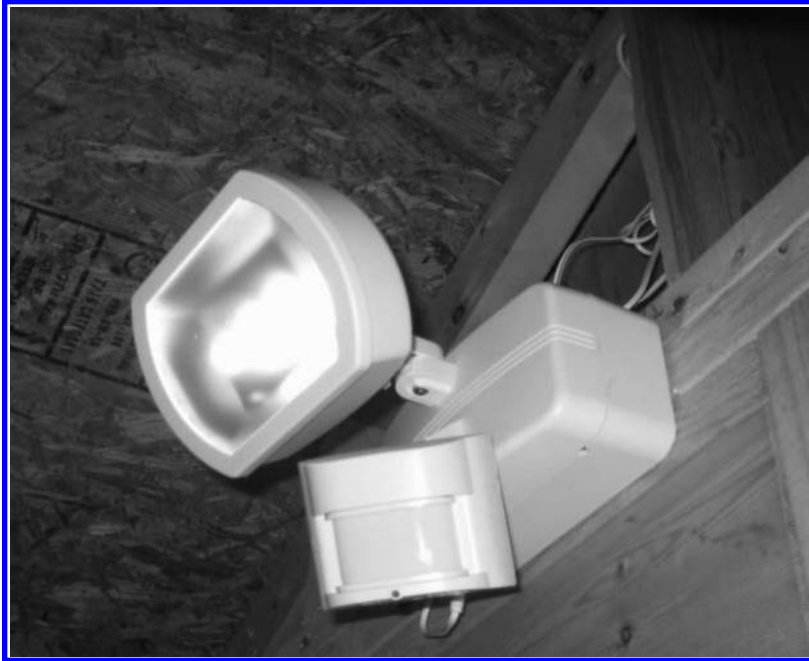
FIGURE E.2 Light-emitting diode floodlight with battery and motion sensor powered by photovoltaic panel. (Courtesy of Parker McGee.)
