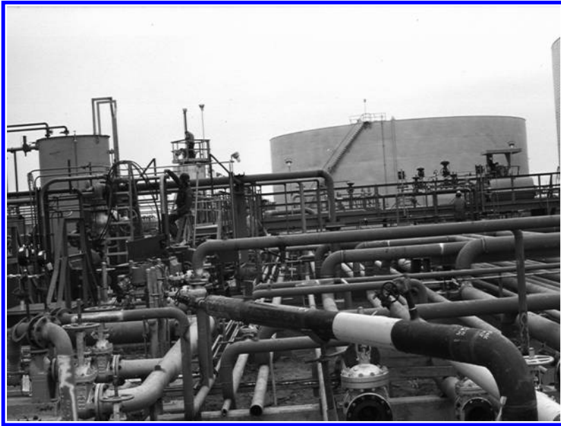
FIGURE 3.1 Photograph of a small section of an oil refinery. (Courtesy of J. K. Yates.)
