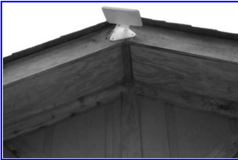
FIGURE E.1 Photovoltaic panel for temporary lighting and storage area lighting. (Courtesy of Parker McGee.)
