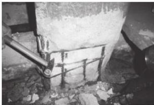
Figure 1. 4 A column steel reinforcement bars after 10 years exposed within a closer area
