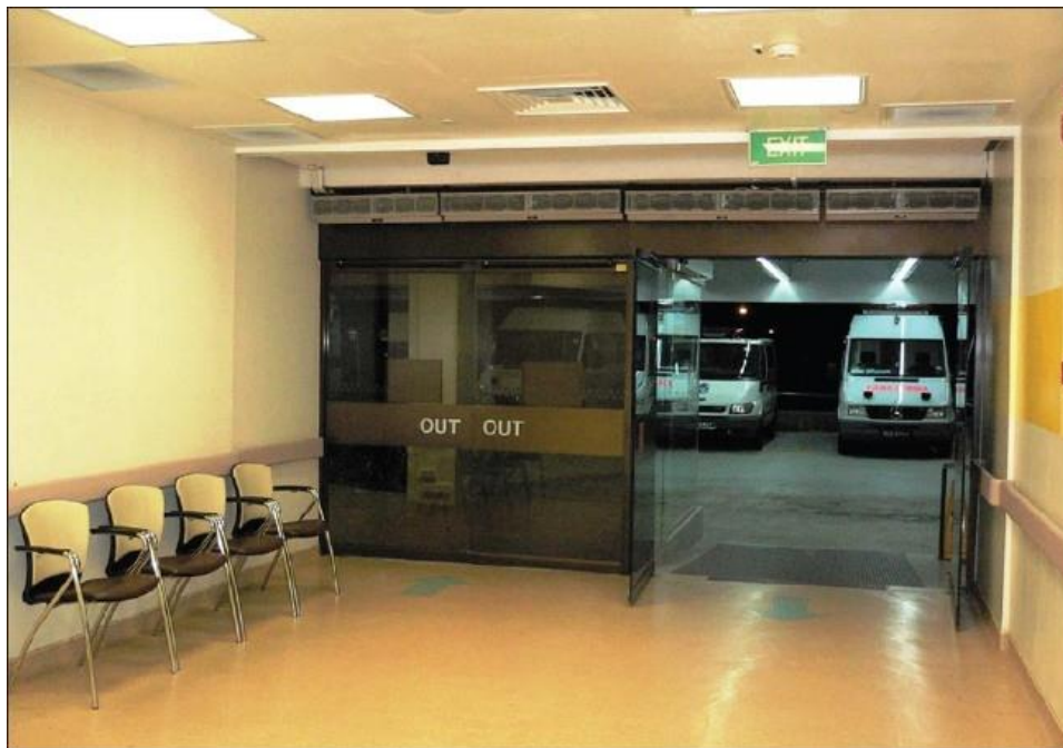
Figure 2 A separate new entrance to the 'fever area' where there is minimal air mix with the other areas of the emergency department
