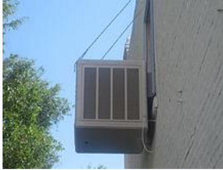
An evaporative cooler
